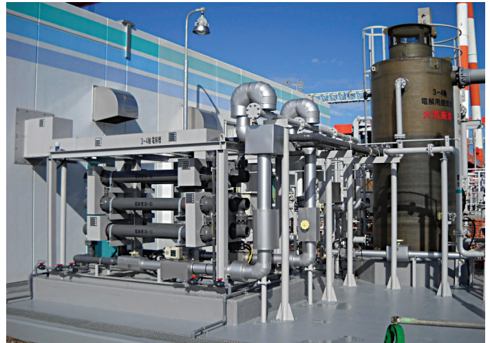
CECHLO-M SWEC 30kg/hr Power Plant in Japan
